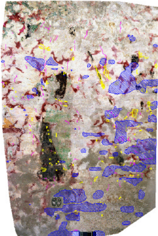
Germany, Königsutter Stiftskirche. Medieval wall painting in the lower storey of the westwork, detail of the Tree of Jesse. Original AutoCAD-mapping of damage phenomena on the base of a rectified color image. Foto: Deutsches Bergbau-Museum Bochum
